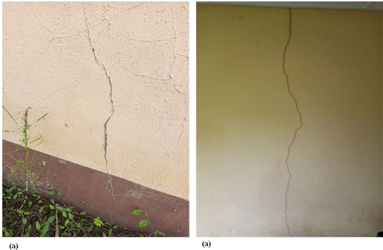
Plate 1 Cracks on the walls of (a) Physics Department building, (b) School of Science building, due to failure of foundation at College of Education (Technical) Asaba.
